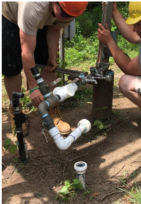
The piping header was reassembled after all in-well work was completed. The pump was then started and an extended flush performed. Pressure is now restored to 60 psi.
