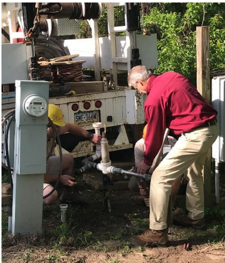
Disassembling the piping header. Co-owner Dave Powell supervised on site for about 2 hours.
