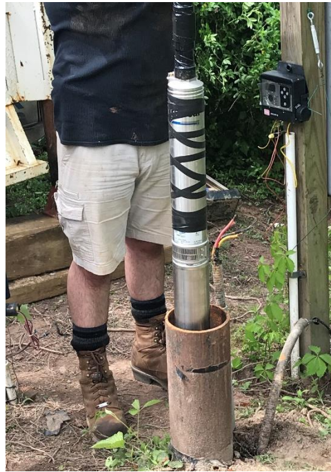
The pump/motor assembly was then lowered into the well casing supported by the first length of PVC pipe (which is rated for an internal pressure of 600 psi).
