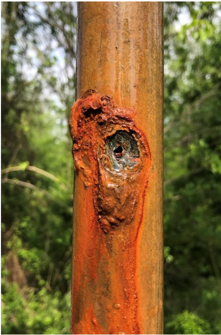
One of roughly half dozen corrosion leaks. These clearly contributed to the 2020 irrigation pressure deterioration.
