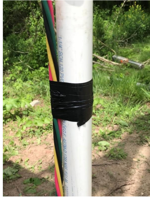
The power cable was taped to the pipe every 8 to 10 feet to prevent chafing against the well casing.
