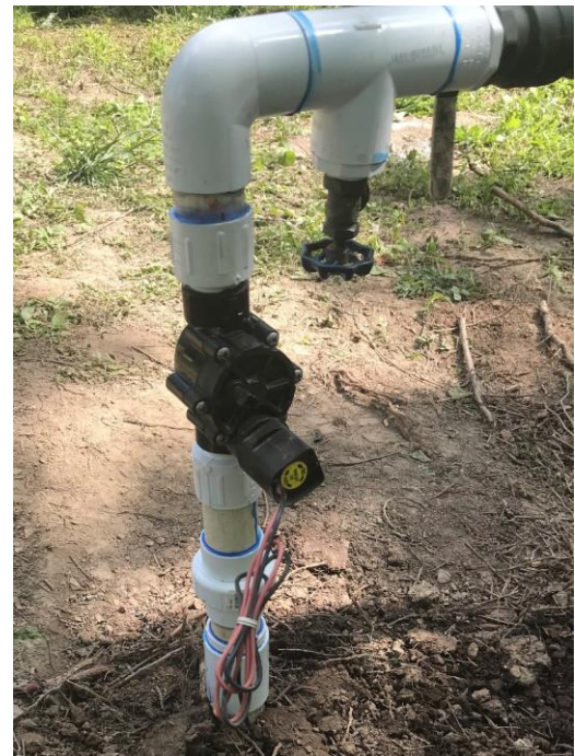
A DC latching solenoid valve was installed in the line to the Sloan irrigation system. It is closed during the day to prevent feeding the leak(s) in the irrigation network. It opens after midnight to provide pressure to the irrigation zones.
