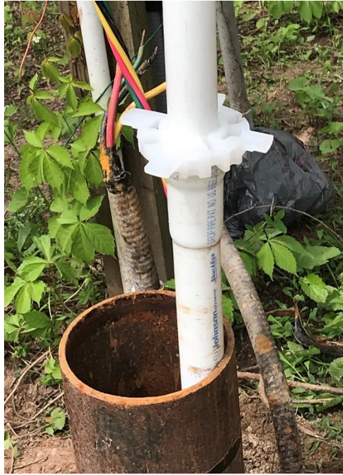
A plastic spacer was snapped onto every length of pipe to keep the pipe string centered in the well casing.
