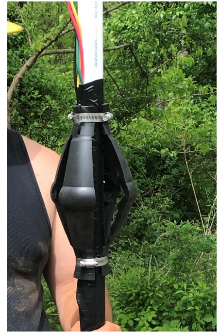
A torque arrester was installed above the pump to prevent twisting of the pipe string when the motor starts.
