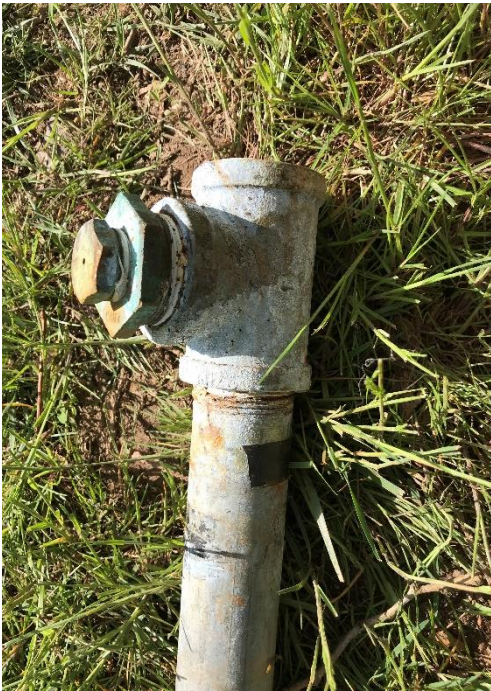
A drain-back valve was discovered in the drop pipe and was reused. This allows water to be drained out of the upper portion of the pipe to prevent freezing.
