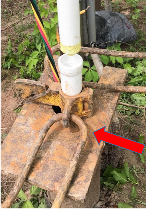
A well pipe clamp secured the first length of 1 1/4" PVC pipe while the next length was threaded into it.
