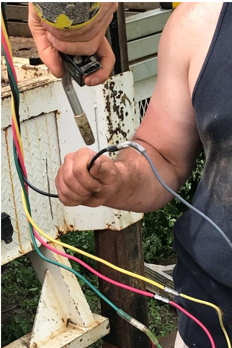
Motor leads were connected to the 4-conductor #10 wire using heat-shrunk waterproof splices.
