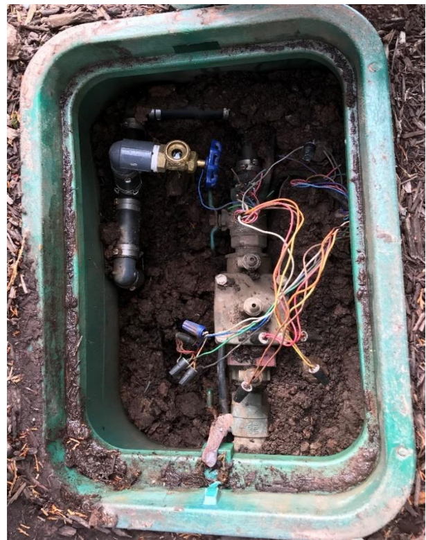
Another subsurface enclosure showing wiring for solenoid zone valves
