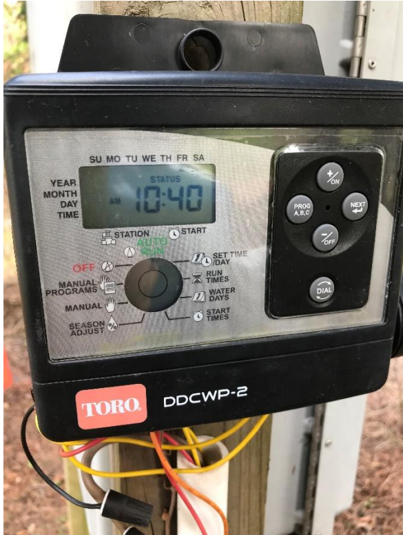
Toro controller operates solenoid valves to either pressurize Sloan Clubhouse irrigation system or to fill Pond 1
