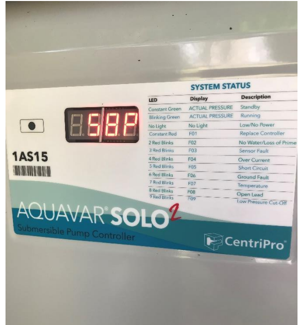
Aquavar controller - varies Pond 1 well pump speed to maintain Sloan Clubhouse irrigation system pressure
