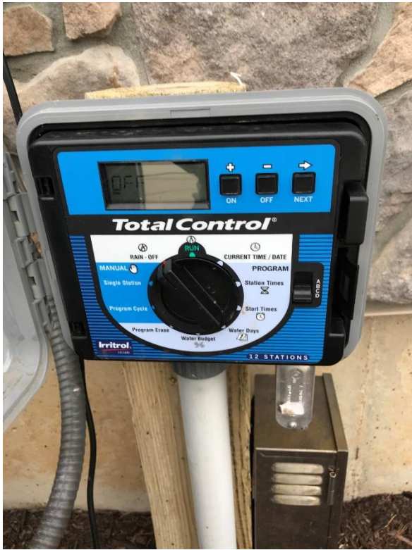
Regency Hills Clubhouse irrigation zone controller – located on west exterior wall
