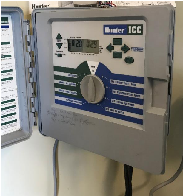
Sloan Clubhouse irrigation zone controller - located on back wall of pool shed
