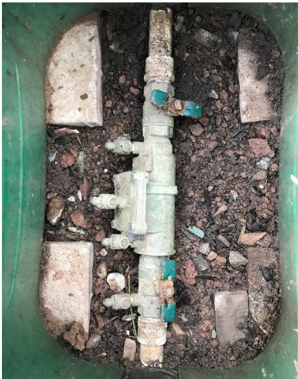
Typical subsurface valve enclosure with shutoff valves (blue handles) & backflow preventer (middle)
