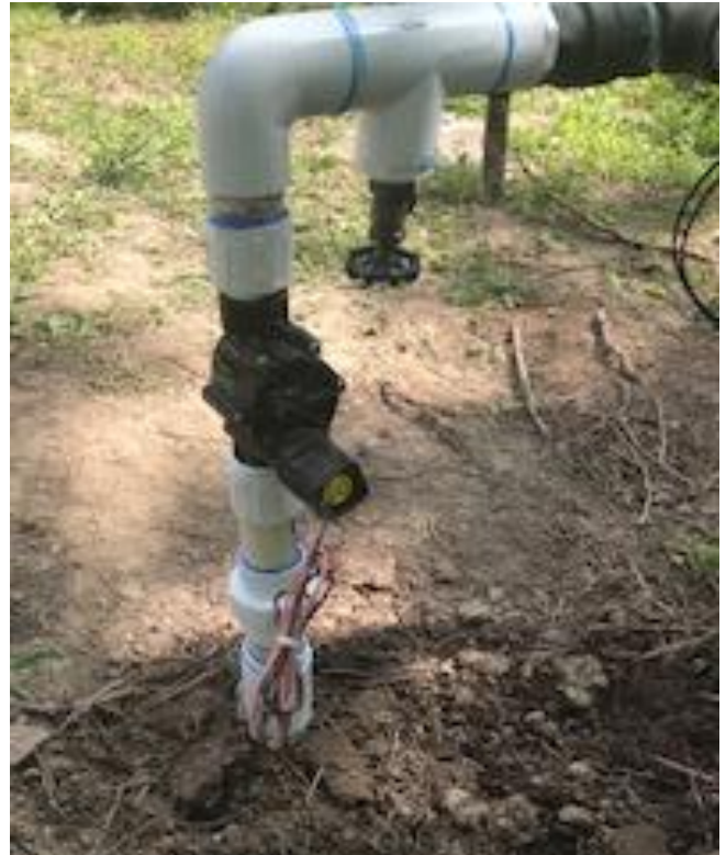
Rain Bird DC latching solenoid valve allows Pond 1 well water to pressurize Sloan irrigation system
