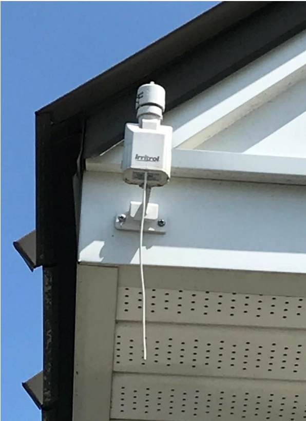
Typical wireless rain sensor - located near each system controller. Suspends watering during rain events.
