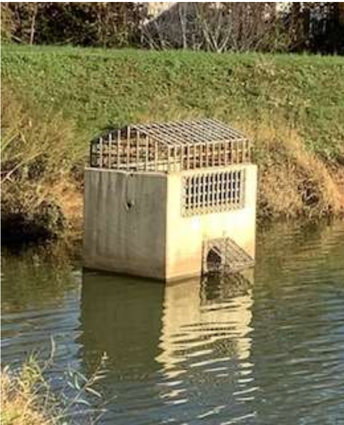
Outlet structure discharges to adjacent variable width conservation easement.
