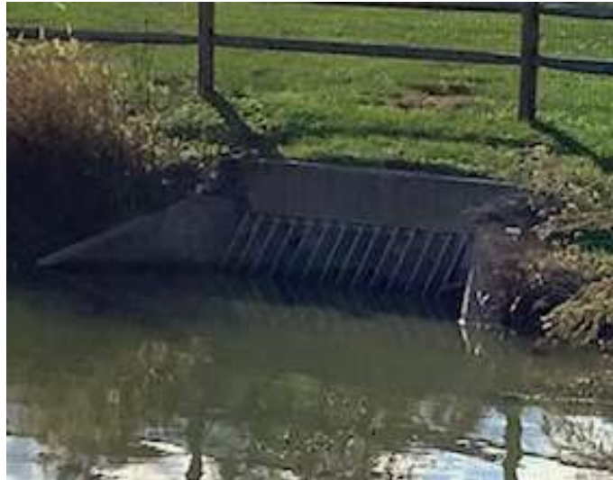
Main inlet structure (one of two) is fed from the Phase 4 storm drains.
