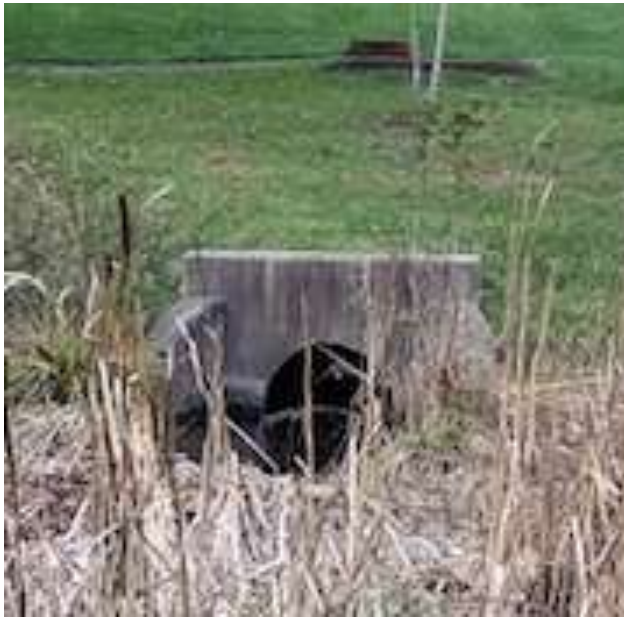
Inlet structure is fed from the Phase 3 storm drains.
