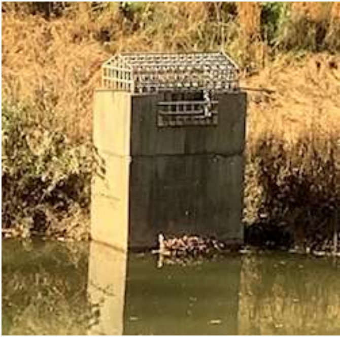
Outlet structure discharges to adjacent wetlands through reinforced concrete pipe.
