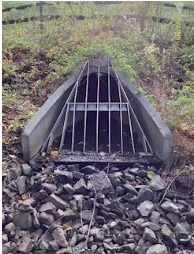
Pond outfall (endwall) is located at the northeast corner of the earthen dam and is similar to those of the other ponds. Riprap in foreground reduces erosion during heavy discharge flow.
