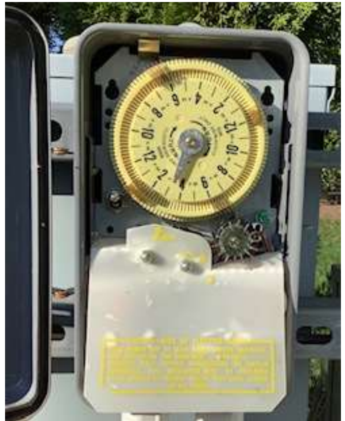
Intermatic timer for well pump is housed in a weather-proof enclosure and is similar to timer at Pond 2.
