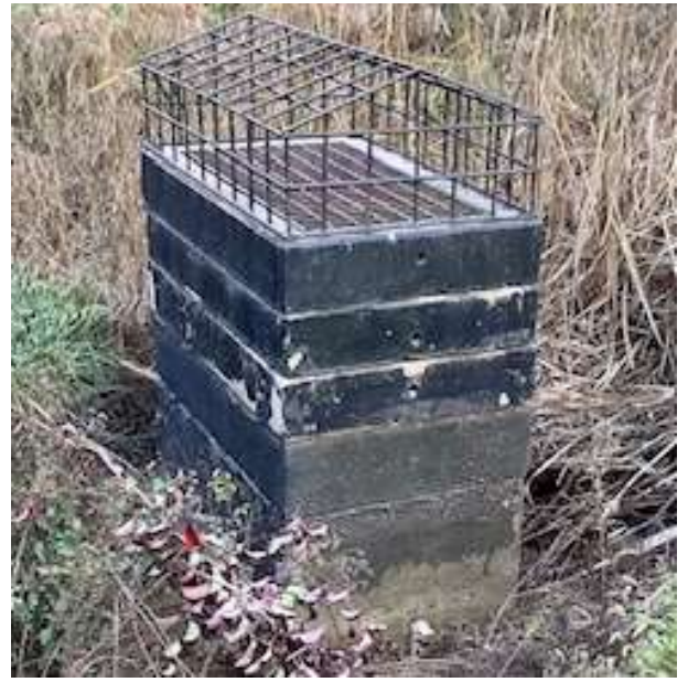
Outlet structure gradually discharges storm water to adjacent wetlands through a 3" diameter bottom orifice. Two sides also have two 1" orifices several feet above the bottom.
