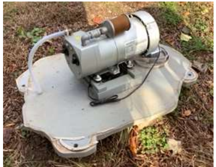
A faux rock enclosure holds the Pond 1 aeration pump. Unit is a Gast rotary vane air pump, model AT05-101-G215DX, 120 volt, 4.7 amp.
