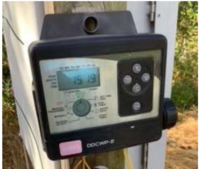
Programmable digital controller located at well site controls amount of make-up water to the pond (as well as irrigation water for Sloan clubhouse).
