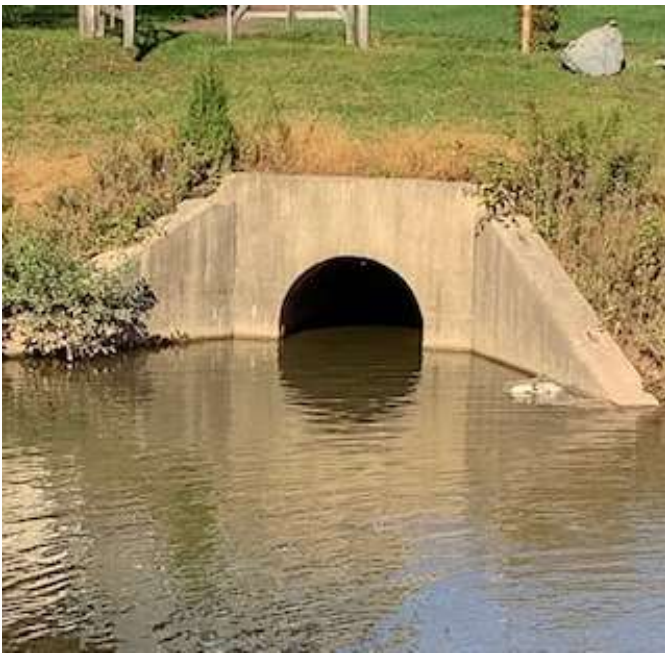
Pond 2 main inlet structure (one of two) is fed from Phase 1 and Phase 2 storm water systems.
