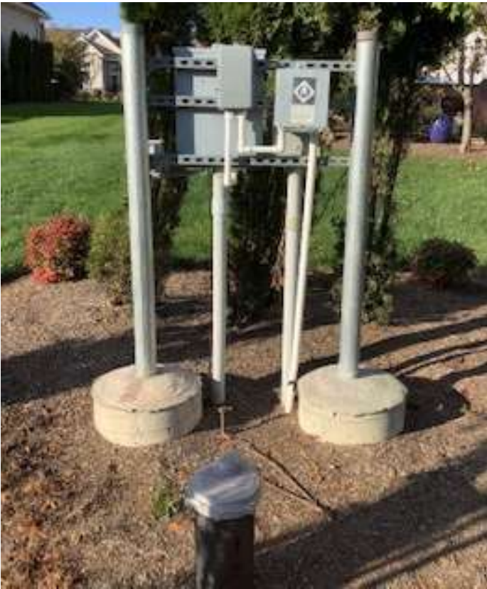
Well site at northwest corner of Pond 4 has electric power panel and well pump controls.
