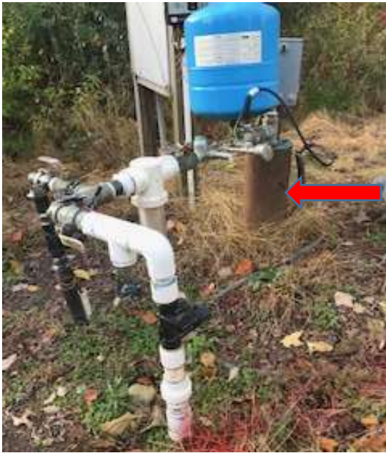
Well discharge equipment header. Arrow denotes exposed portion of the steel well casing.
