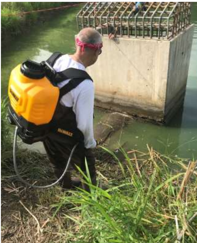
The ground-out joint was flushed with clear water from a backpack sprayer.
