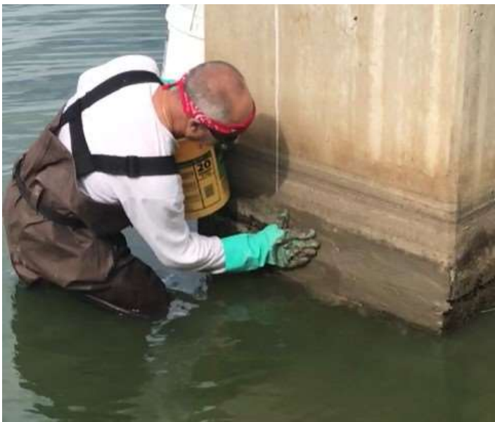
After hand mixing the cement with water Ed worked quickly to stuff the joint before the material set up. The first pre-weighted packet of grout was enough to cover the area shown.
