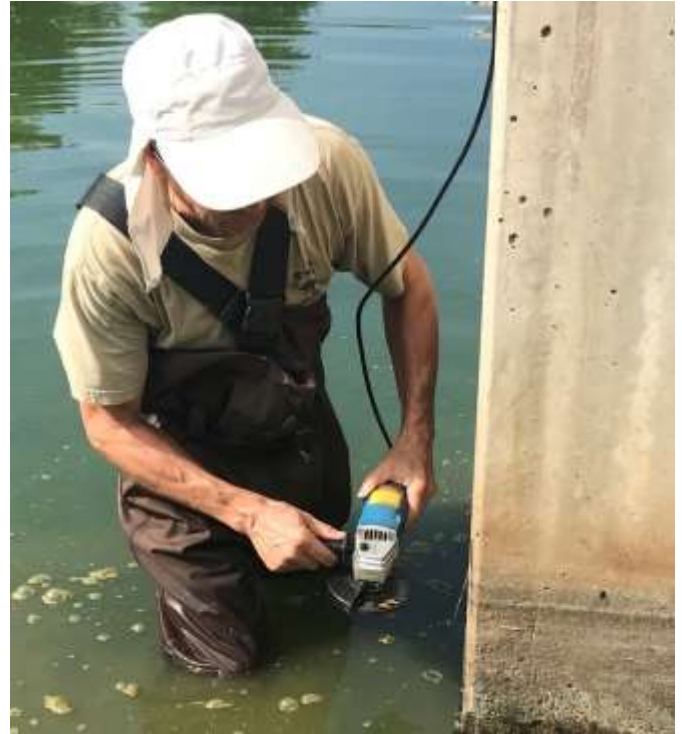
After wire brushing the joint, an angle grinder was used to clean out old grout and provide a cavity for the hydraulic cement.
