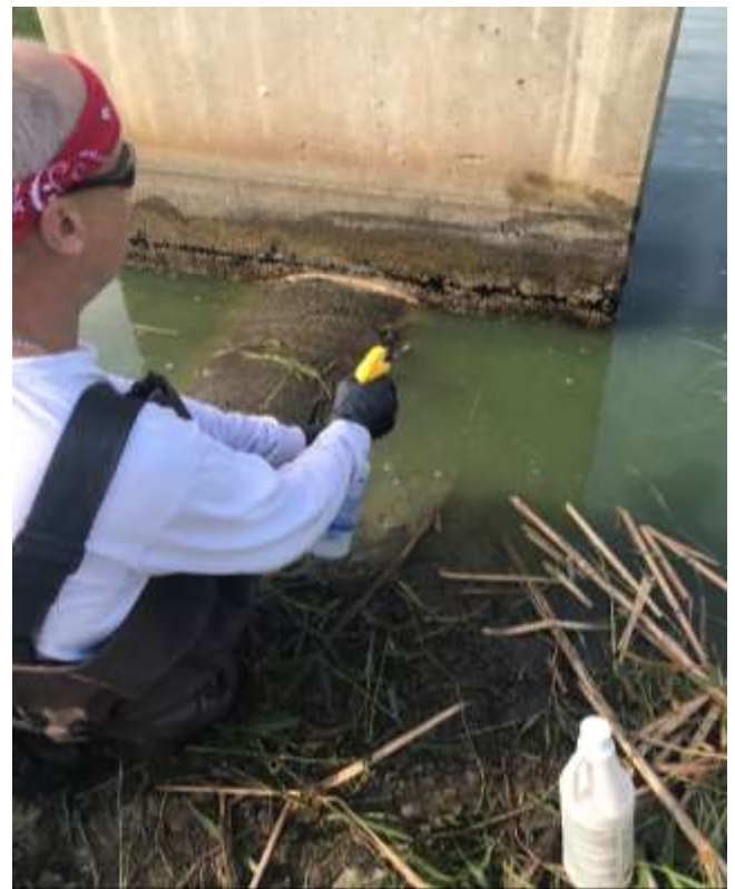
Acid etching the joint with dilute hydrochloric acid dissolved contaminants, creating a better bonding surface.
