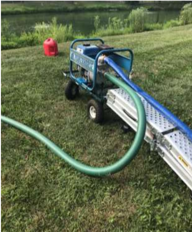
The pond level was lowered using a gasoline-powered, 2" trash pump rated at 130 gallons per minute. It was discharged (blue hose) into the drainage easement north of the pond.
