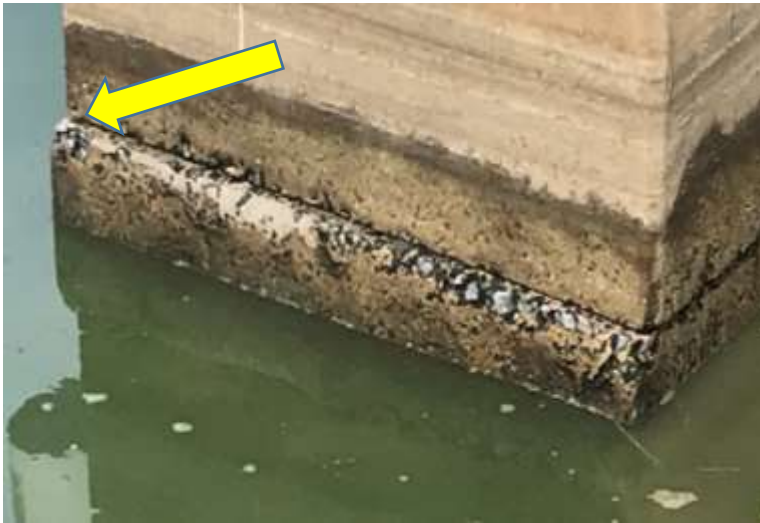
After rinsing out the acid, neutralizing the surface with ammonia and a final water rinse, all four sides of the joint were ready for grouting. Note the misalignment of the stacked sections evident at the left hand corner of the structure.
