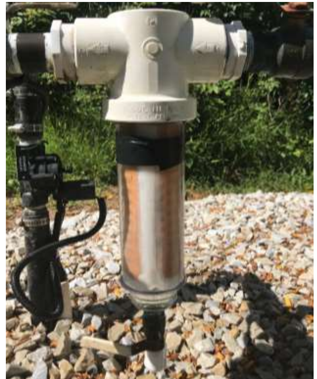
The grit filter prevents particles from flowing downstream and plugging the sprinkler nozzles.
