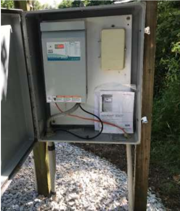
The Aquavar well pump controller is mounted in the upper left corner of this weatherproof cabinet.
