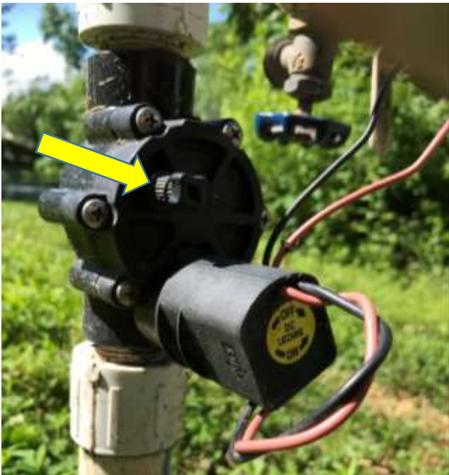
The two Rain Bird solenoid valves are controlled by the Toro unit but can also be operated manually using the knurled control knob (CCW to open).
