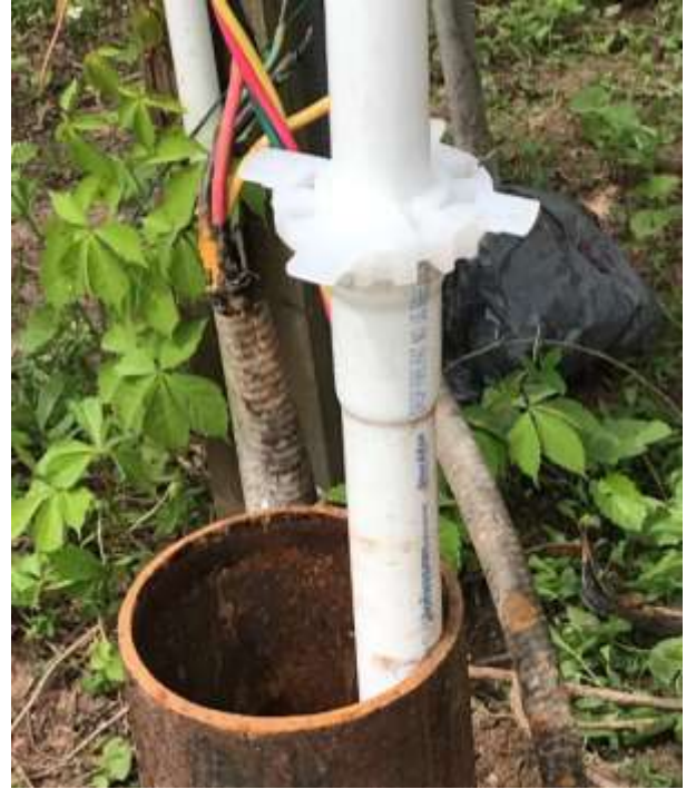
A plastic spacer placed on each 20' section of PVC drop pipe keeps the pipe string centered in the 6 inch diameter well casing.
