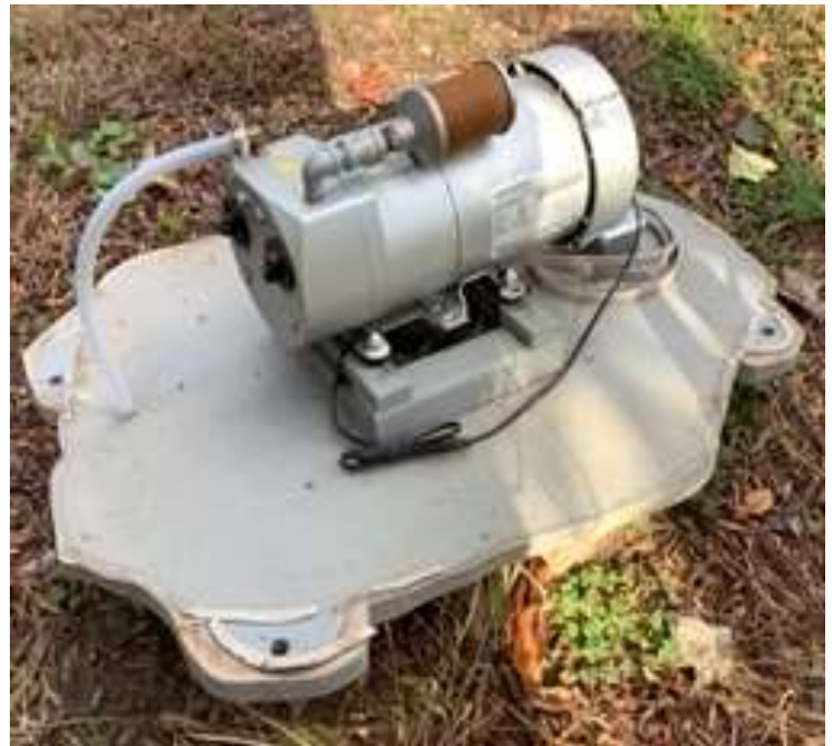
Around-the-clock pond aeration is supplied by the Gast air pump, which is housed in a faux rock enclosure.
