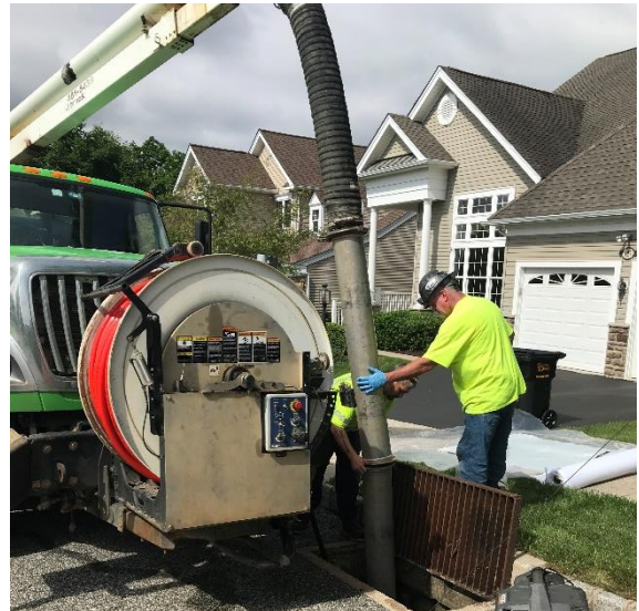
Connecting sections of vacuum line prior to jet cleaning the damaged RCP section. Note the reel of high pressure hose.
