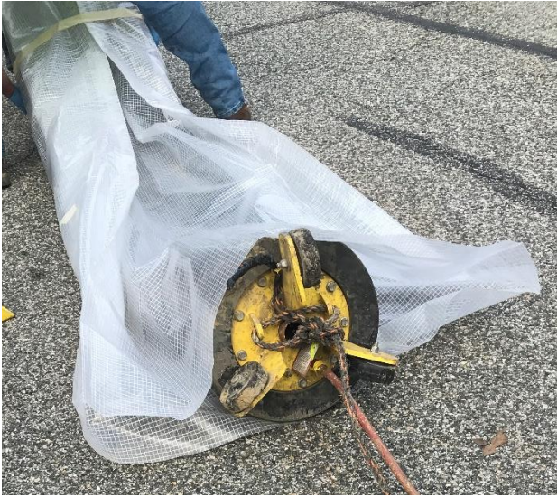
The packer is roped at both ends and wrapped in plastic to prevent the resin from contacting the rubber bladder. Note the red air hose used to pressurize the packer.
