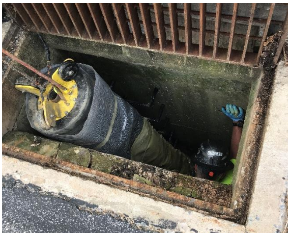
One crew member lowers the packer into the inlet structure, a second guides it into the pipe and the third pulls it into position from the downstream inlet.
