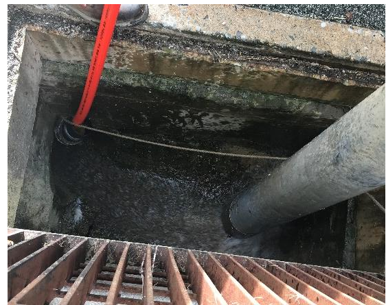
The cleaning hose progresses up the pipe (to the left) while the vacuum system extracts spent wash water.
