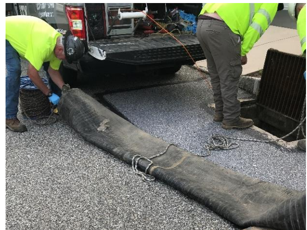
The inflatable rubber packer is prepared for deployment into the stormwater line.
