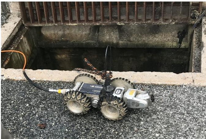
Once the section of line is cleaned a camera-crawler is used to confirm the exact location of the defect.
