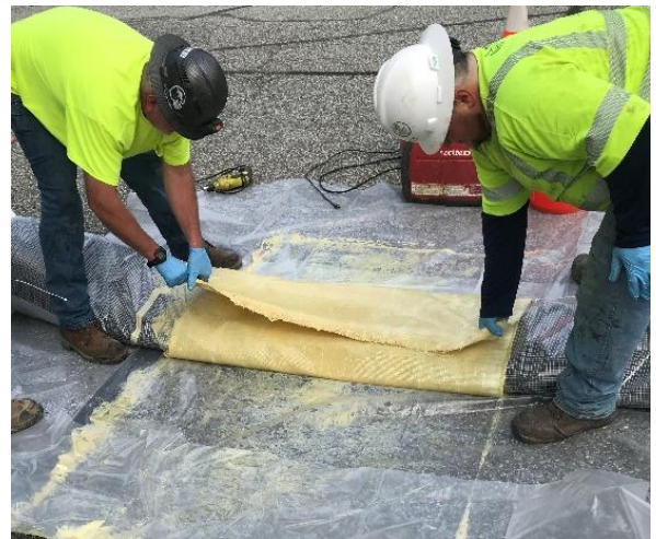
The resin-impregnated sleeve is then wrapped around the packer and secured with plastic zip ties.
